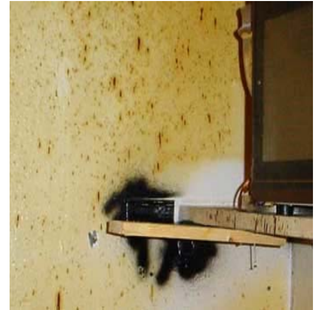
Chemical staining on interior walls
