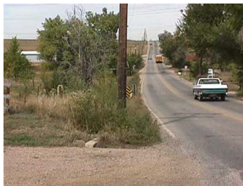
Inadequate shoulder clear zone
