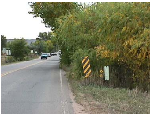
Vegetation protruding into travel lanes
