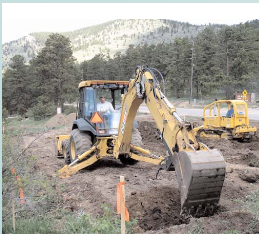
Breaking ground at the Dog Off-Leash Area near Elk Meadow Park in Evergreen.
